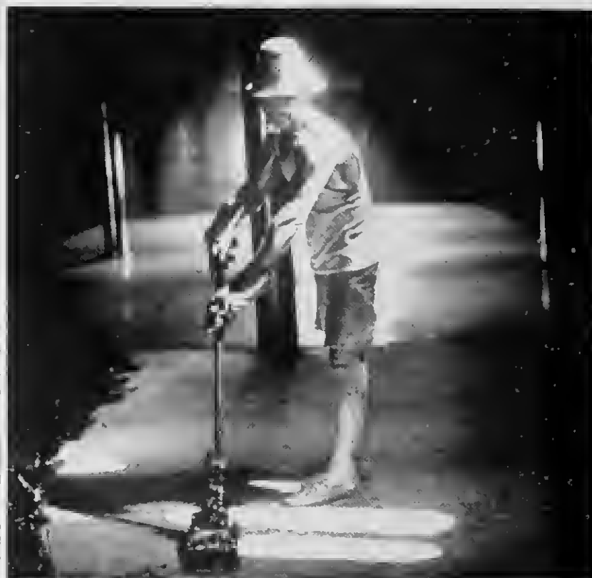
PICTURED in a shaft of sunlight pouring through a hole in the top, a workman spreads asphalt on the floor of a tank now being built on Seroe Pretoe. Soon this floor will be covered by 1,500,000 gallons of water.
